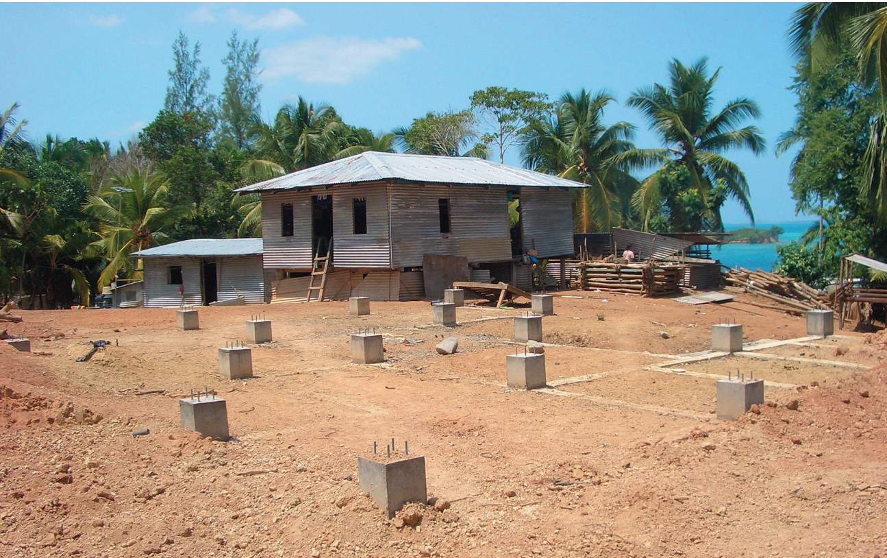
Photo 5: Concrete foundations laid for the construction of permanent shelters in Nancowrie Island. The use of non-traditional material for the construction remains contested, besides the fact that after four years the progress made remains inadequate
